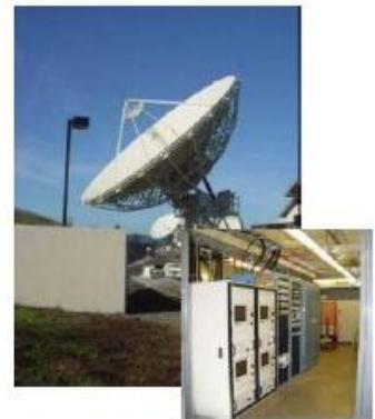
4 Ground Earth Stations
