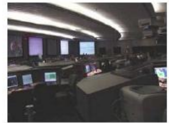
2 Operational Control Centers
